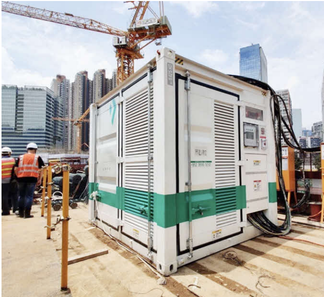
Electric generators for improved site safety, air quality, and reduce operational carbon and noise pollution.
