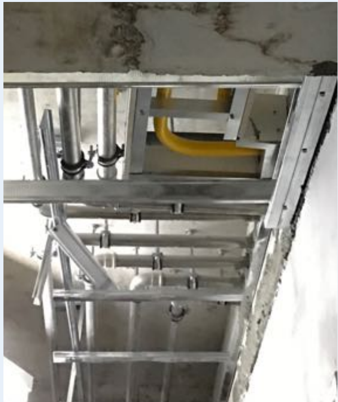
Figure: Sample of Concealed Services in the Ceiling Space
