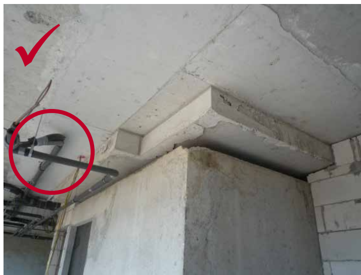
Running insulated air-con drain pipes at ceiling and connect to a separate stack pipe
