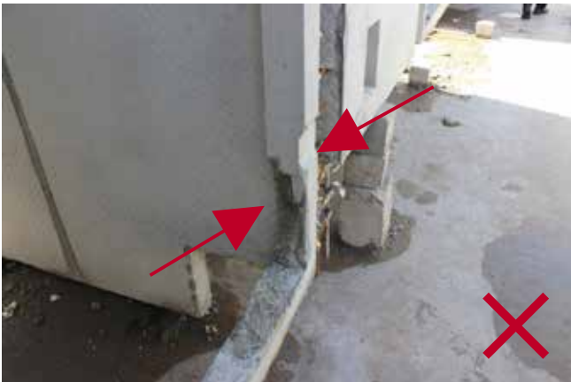
Damage after stripping formwork
