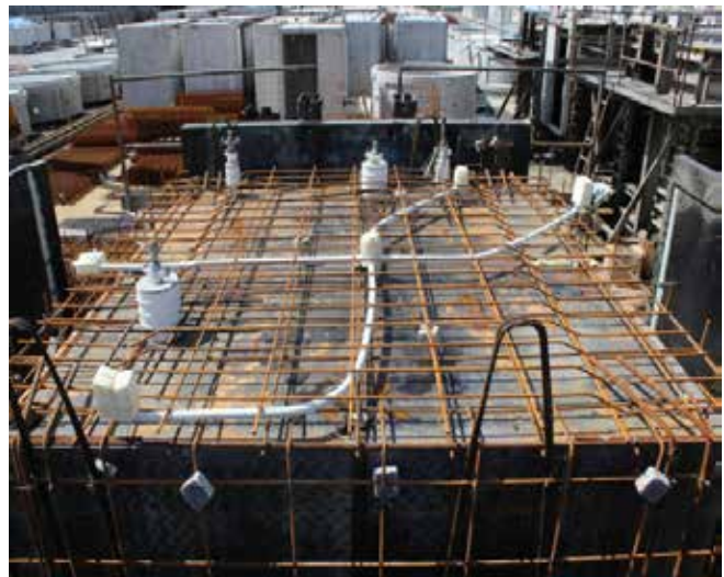
Embedded M&E services on slab
