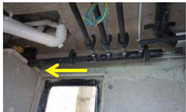
Air-con drain pipe connecting direct to stack
