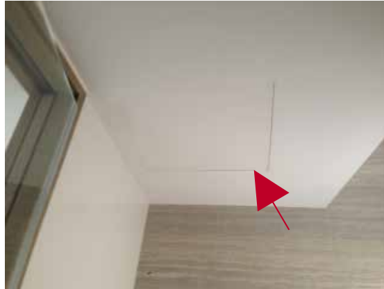
Ceiling Access Panel Location
