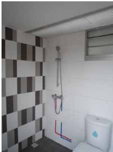
Demarcation of hot and cold water supply by coloured tapes
