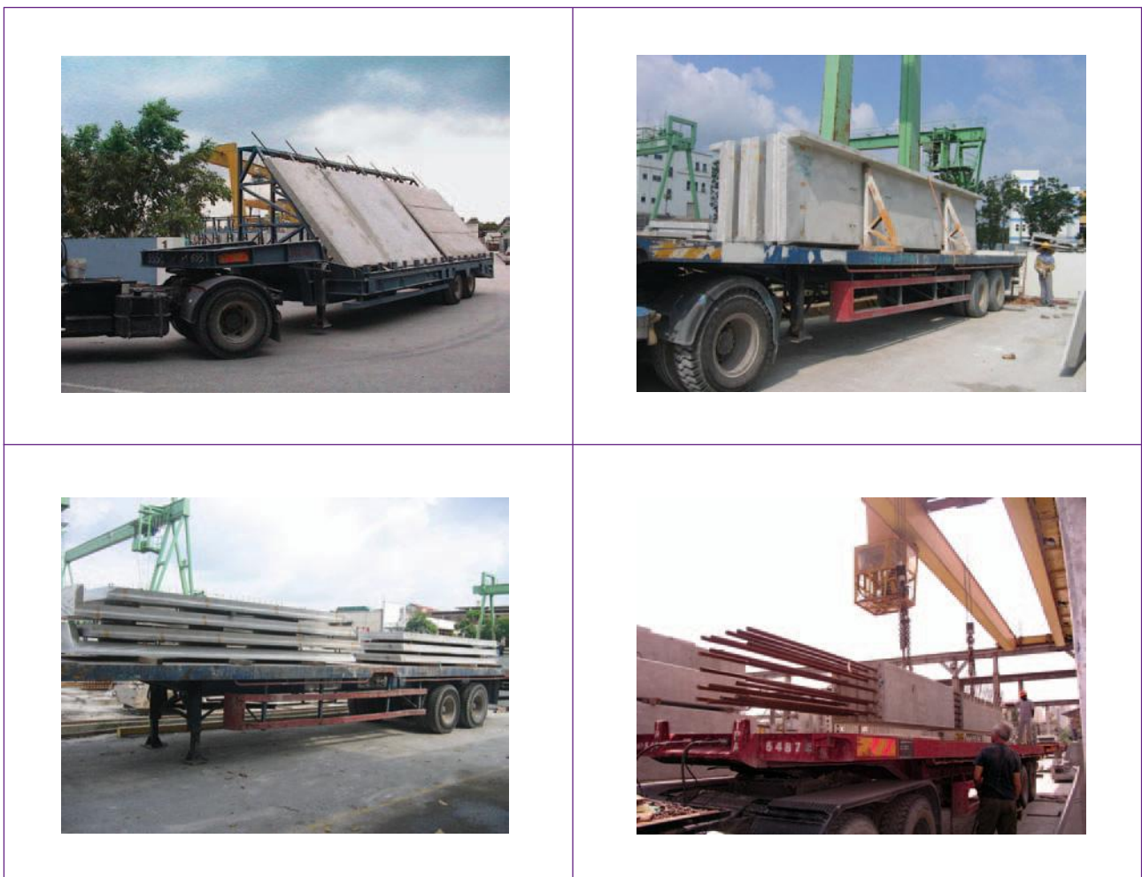
Figure 4.1 The manner of delivery will depend on the type, dimension and weight of the precast elements
