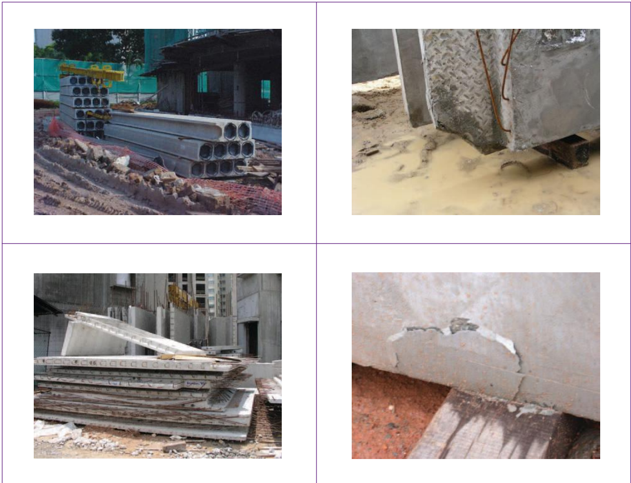
Figure 4.11 Examples of improper storage and stacking methods
