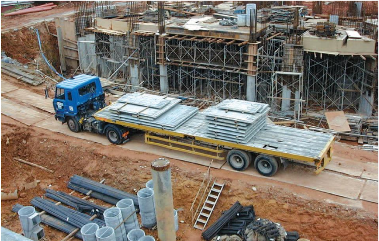
Figure 4.3 Precast elements should be adequately fixed and secured to pre-empt movement or accidental spillage during transit
