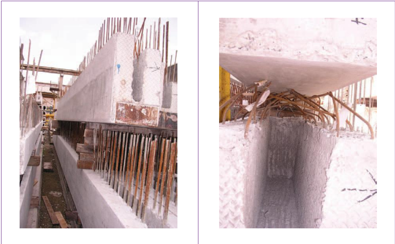
Figure 2.4 Long projecting bars may pose storage and handling problems
