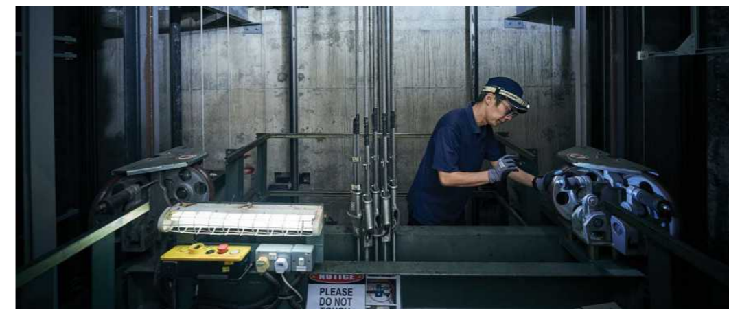
Lifts equipped with remote monitoring and diagnostics capabilities enabled predictive maintenance and improved lift performance.
