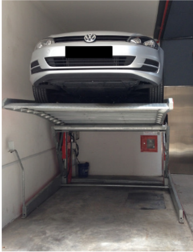
Figure B1 – Standalone lifting system for a single car within a building
