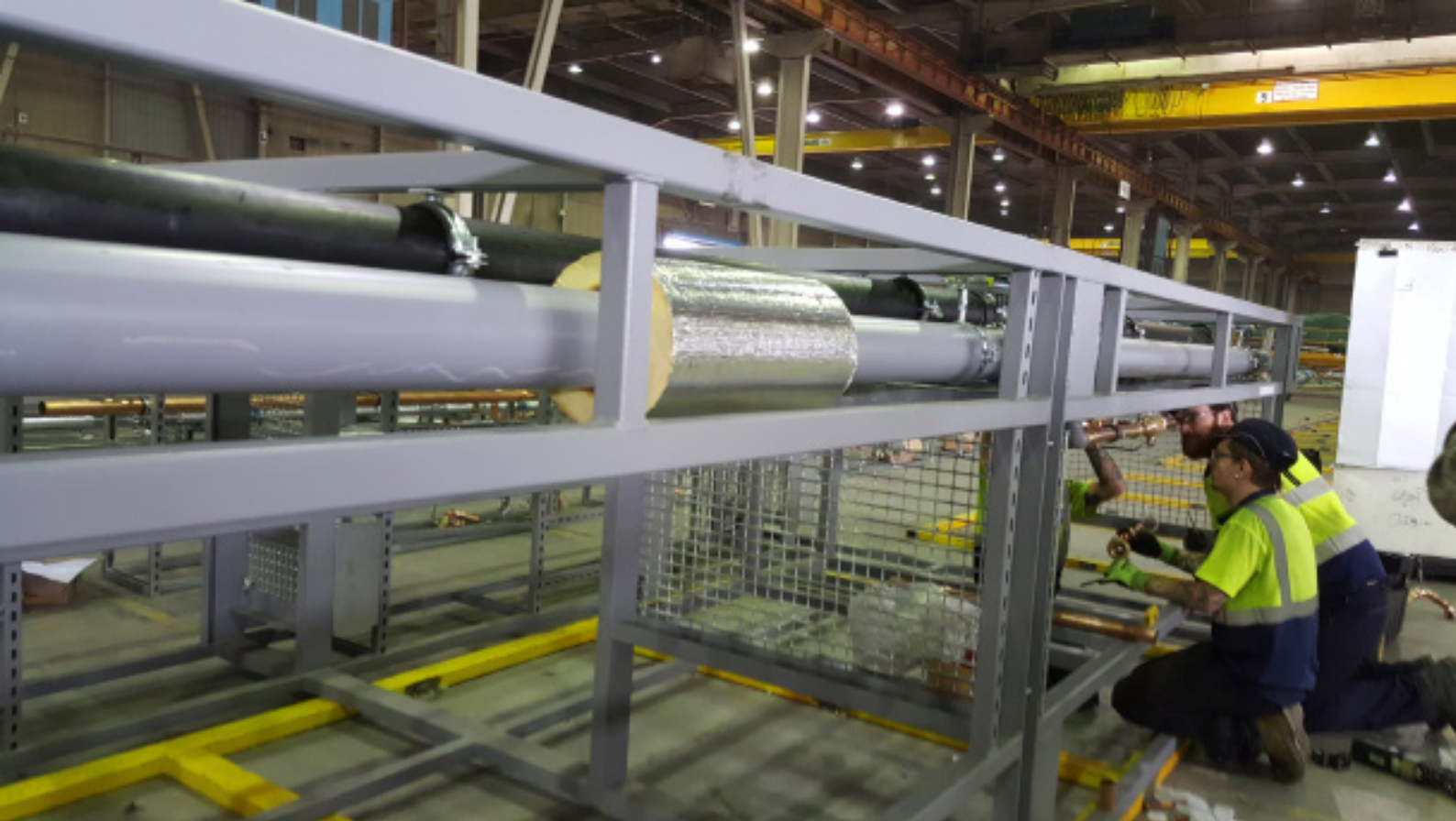
Figure 11: Ensuring quality control at the MEP factory ( Photograph courtesy of Crown House Manufacturing, United Kingdom )
