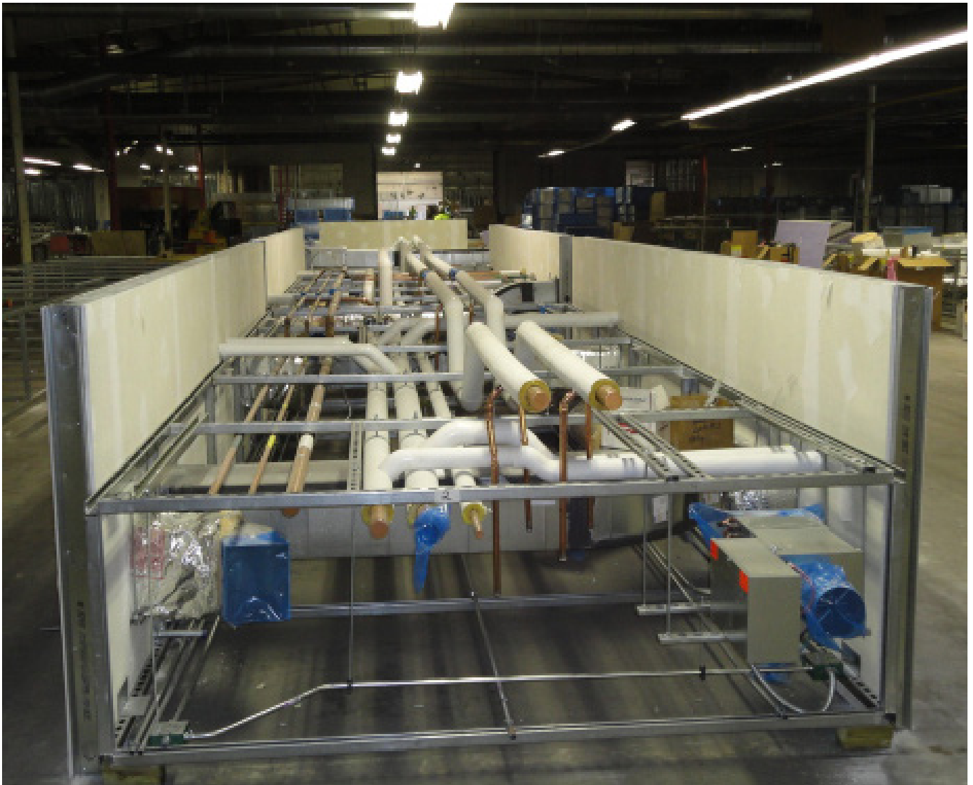
Figure 13: A horizontal ceiling module integrated with drywall partition wall to facilitate installation in tight working space.
