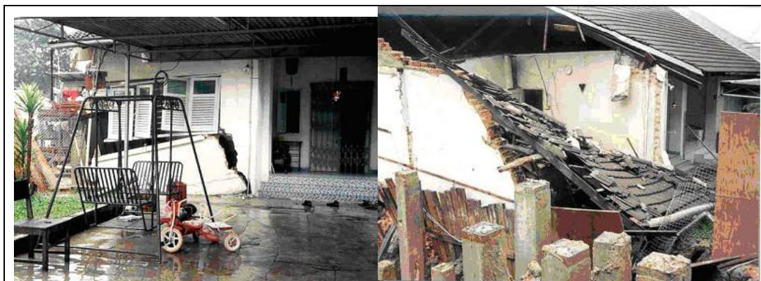
Figure 2: Cracking and collapse of adjacent single-storey house .
