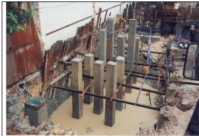
Figure 1: Shoddy timber planks to support excavation for pile cap
