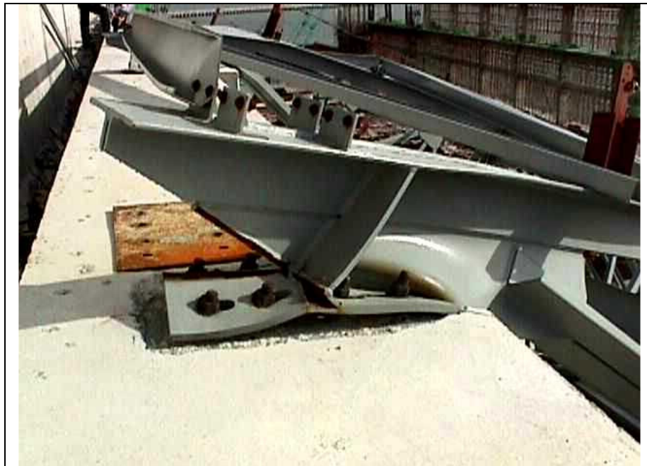
Figure 3: Knee-joint at support. The angle cleats to hold purlins were not continuous.
