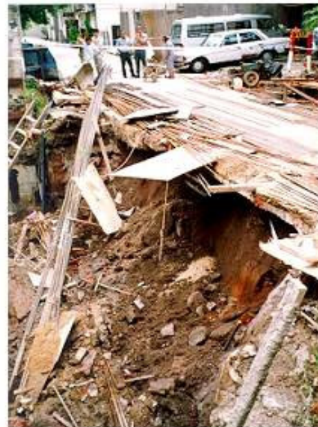
Figure 2: Collapsed part of excavation
