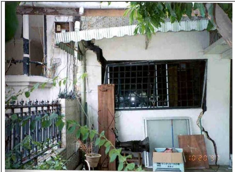
Figure 2: adjacent unit affected by tilt of the corner terrace
