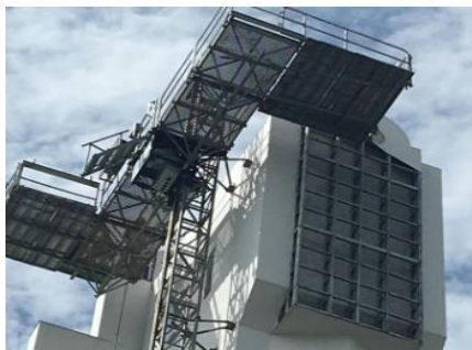
Image 1: Fallen Board Cladding
