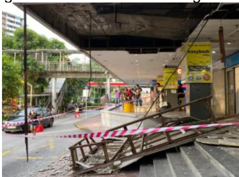
Image 3: Collapsed Exterior Ceiling
