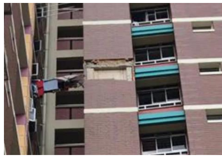
Image 2: Fallen Brick Facade
