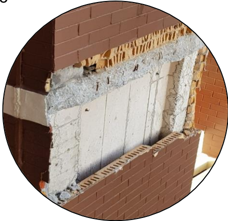
Fallen brick facade
