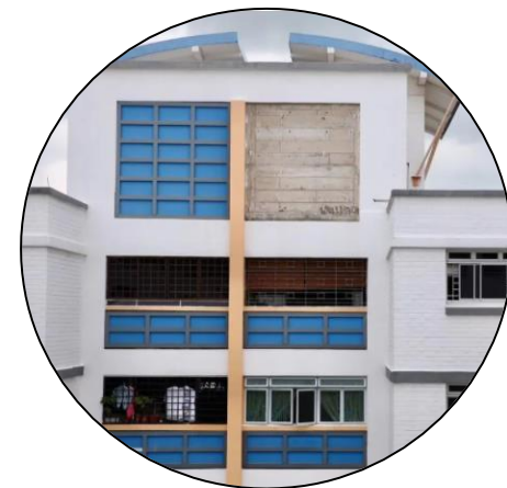
Dislodged metal cladding
