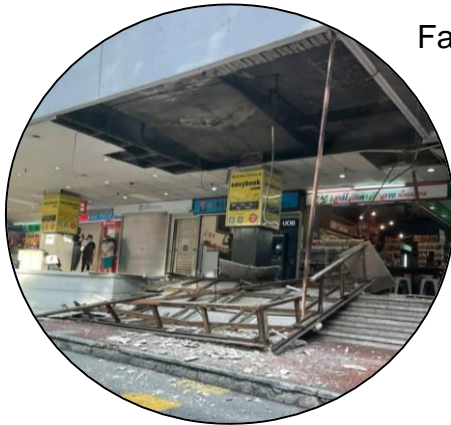
Collapsed exterior ceiling
