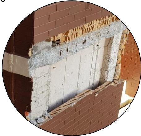
Fallen brick facade
