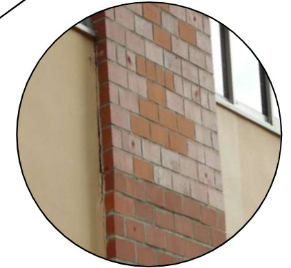
Bulging brick facade
