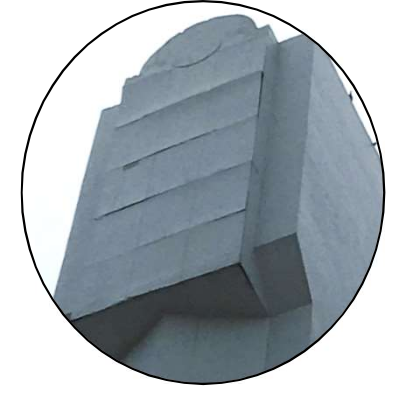
Bulging board cladding
