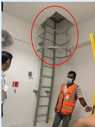
Figure H—VIII: Locked-entry cat ladder / hatch doors; with signage to indicate maintenance area
