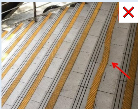
Figure E—XXVIII: Unacceptable nosing finishes - Adhesive nosing tapes
