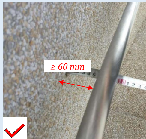
Figure E—XVIII: Clear space from rough wall surface (Min. 60mm wall gap)
