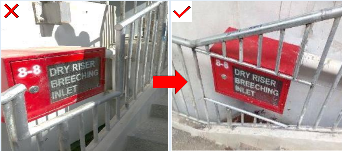
Figure E—XIX: Non-continuous handrail due to MEP fixture
