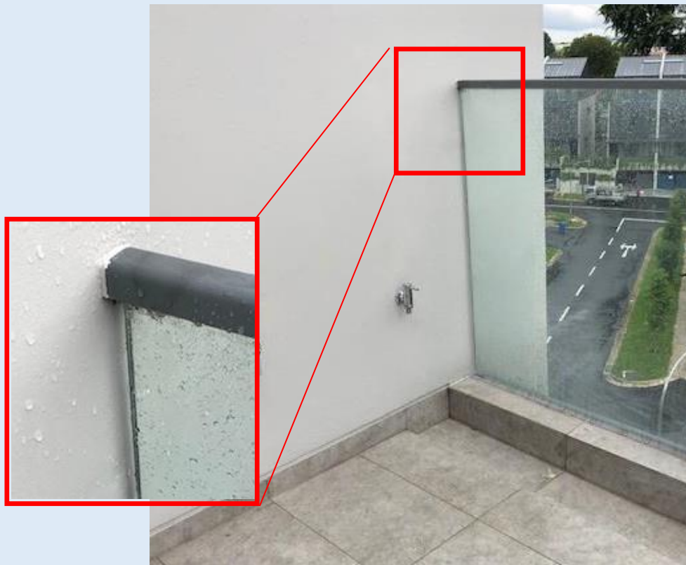
Figure H—XXXV: An example of glass barrier with continuous rail fix to top edge of glass
