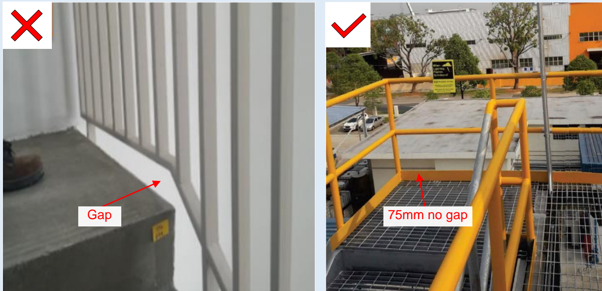
Figure H—XXV: No gap at 75mm from FFL is applicable to M&E areas
