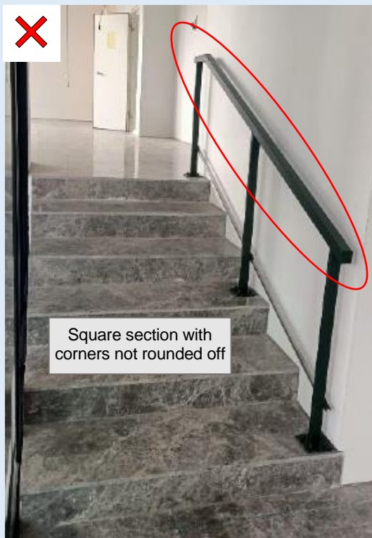
Figure E—XV: (Photograph 1) Unacceptable handrail profile
