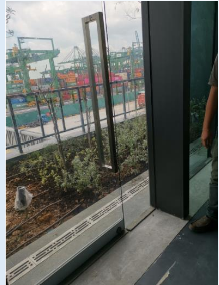
Figure H—VI: Accessible door opening to the maintenance roof through common space
