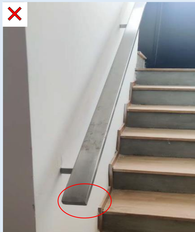
Figure E—XVI: (Photograph 2) Unacceptable handrail profile
