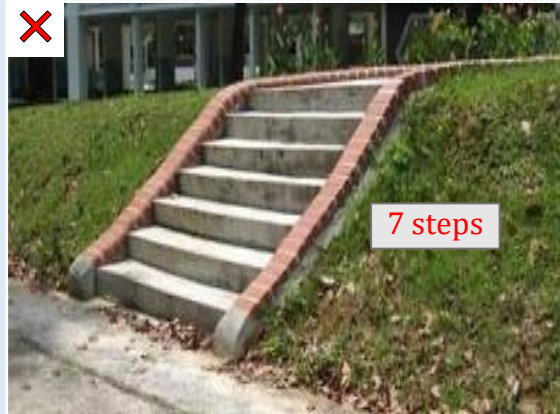
Figure E—XI: Photos from site inspections that depict staircase which are not provided with handrail
