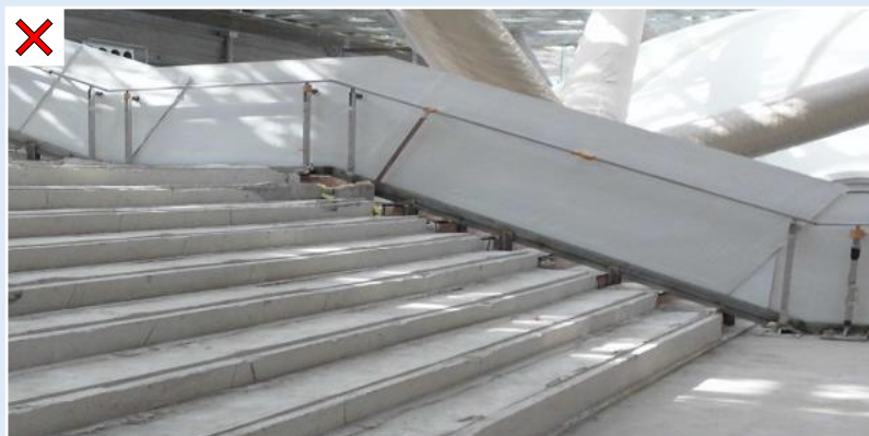
Figure E—VI: Incomplete finishing work
