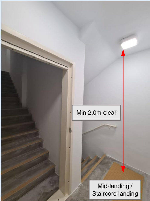
Figure C—XV: Headroom at staircase mid-landing with projection of light fixture
