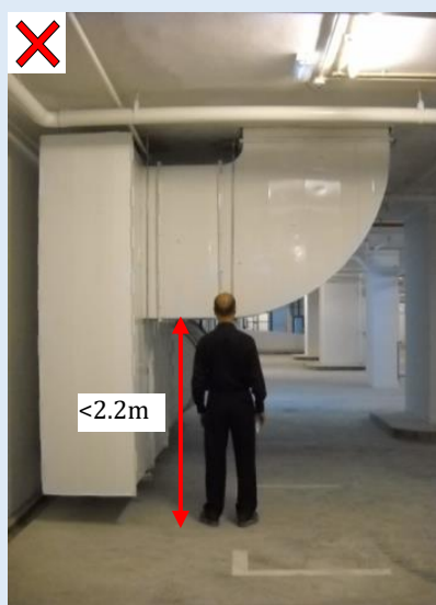
Figure C—X: Headroom non-compliances at the parking lot
