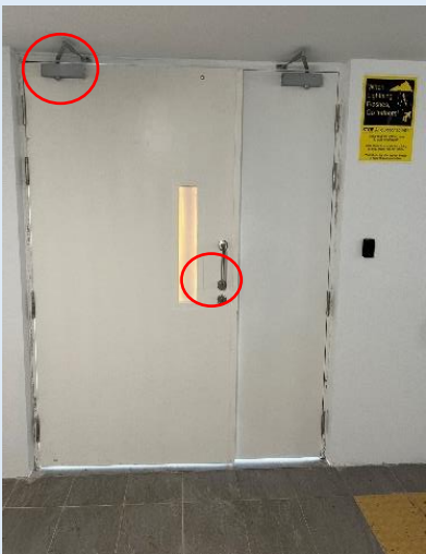
Figure H—VII: One-way lock and self closing door / gate; with a signage to indicate maintenance area
