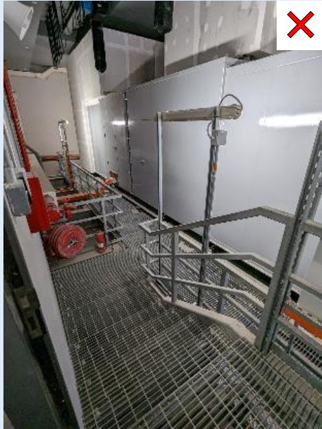
Figure E—XXIII: No nosing provision at maintenance areas
