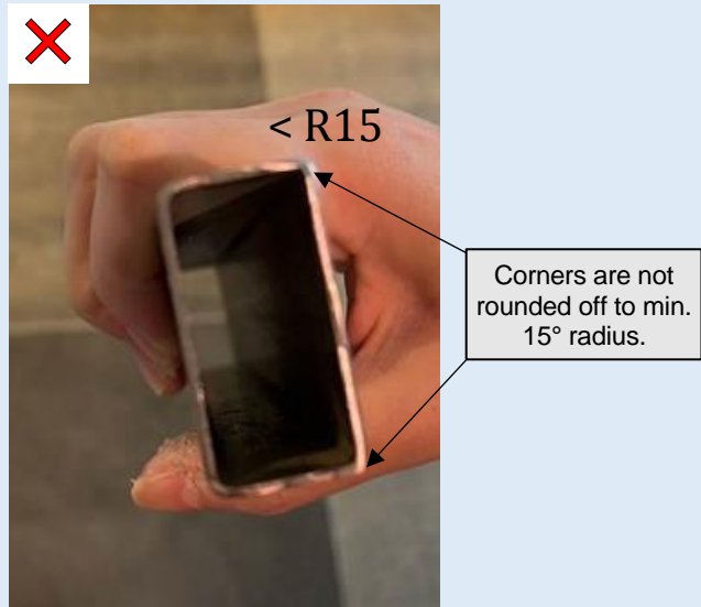
Figure E—XIV: Unacceptable handrail profile with sharp corners
