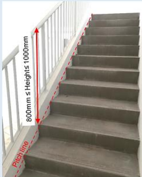
Figure E—XII: An example on the measurement of height of handrail from pitch line
