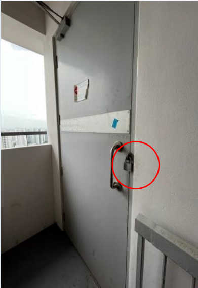
Figure H—IV: Door with padlock or a padlock gate to a maintenance area
