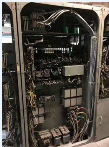
Figure 3: Outdated Lift Controller
