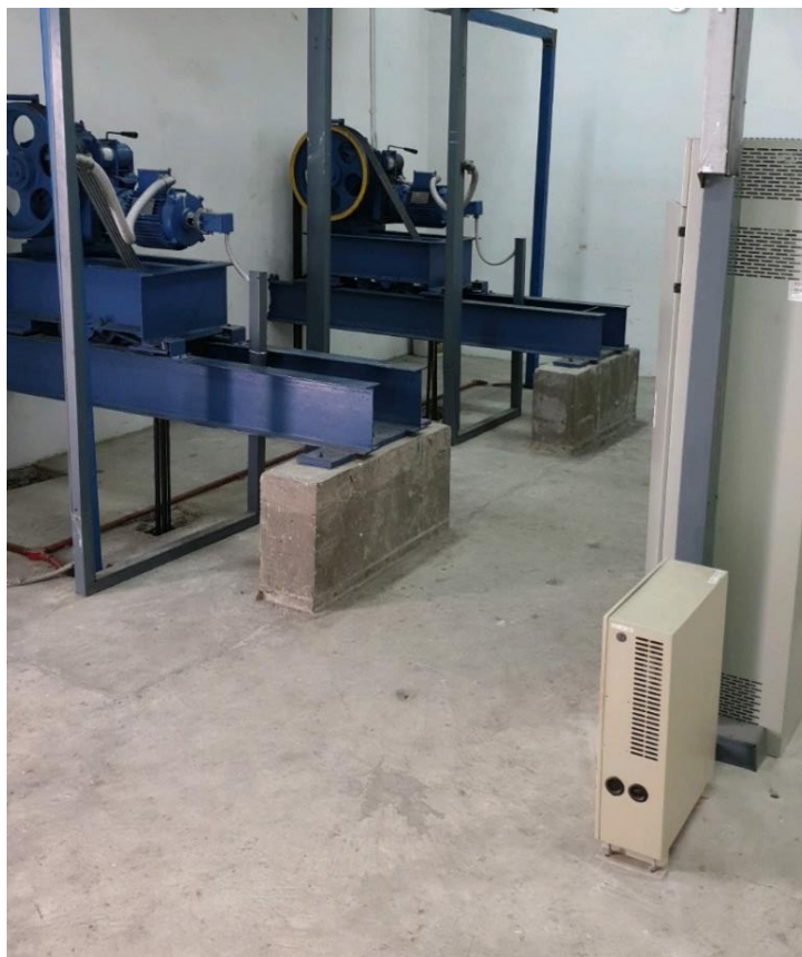
Clean and tidy motor room
