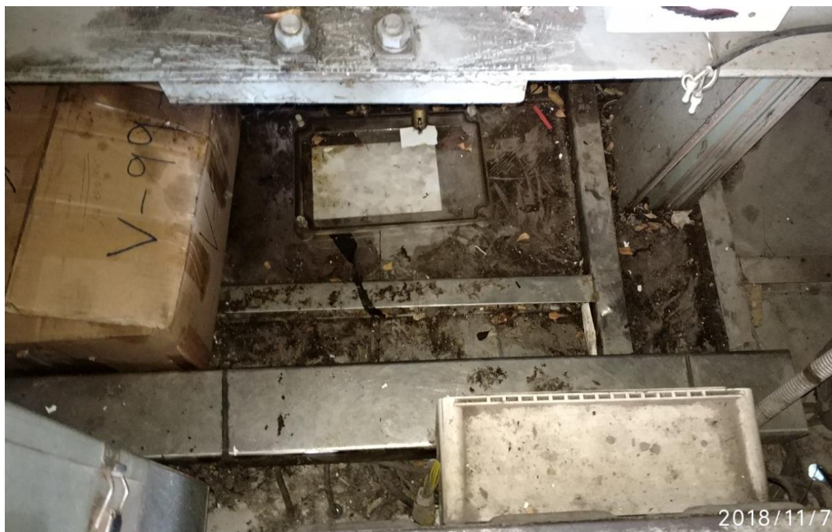
Poor housekeeping of lift car top
