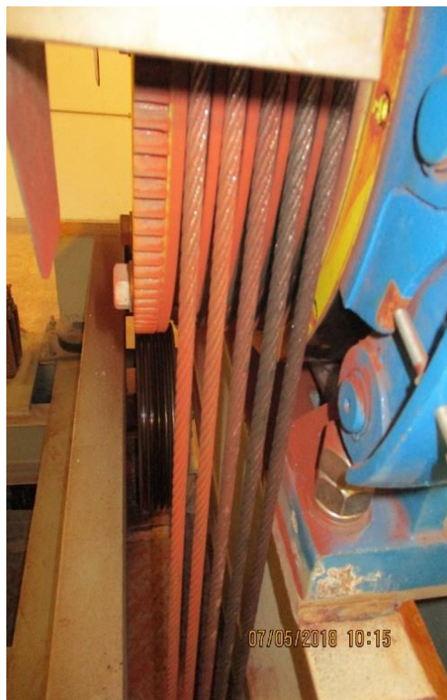
Rust on lift machine
