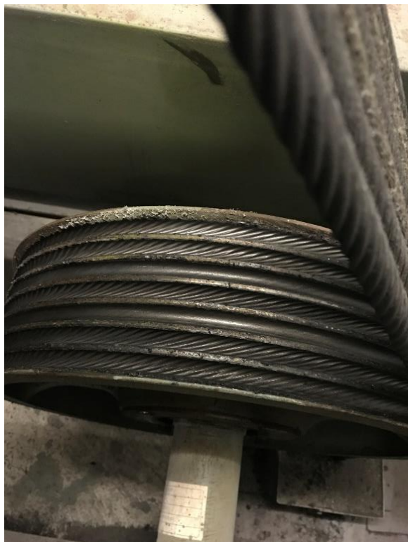
Excessive wear on deflector sheave
