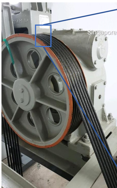
Lift drive machine
