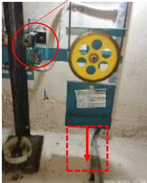
Governor rope tensioning sheave
