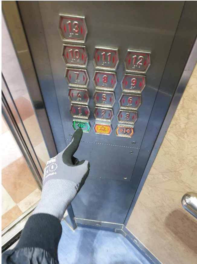
Door open button check - lift car
