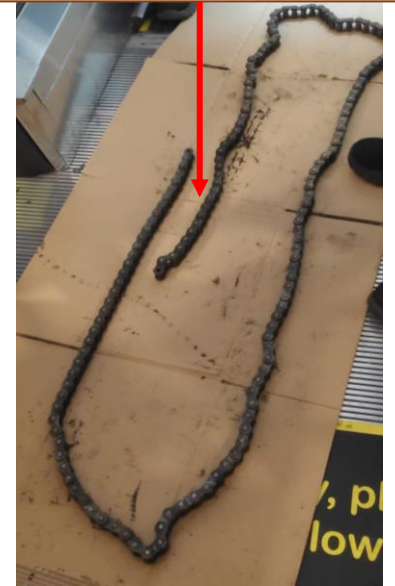
Broken Handrail Chain
