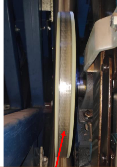
Worn out Handrail Sheave.
