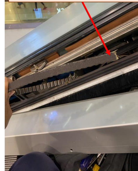
Broken Handrail Drive Belt
