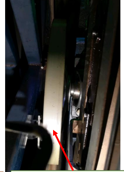
New Handrail Sheave.
