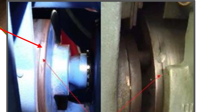
5. Contaminated Brake Drum (Oil Stain)
