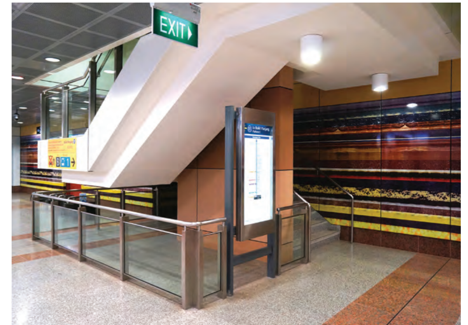
Photo: A guardrail to warn and keep users away from areas with low headroom
