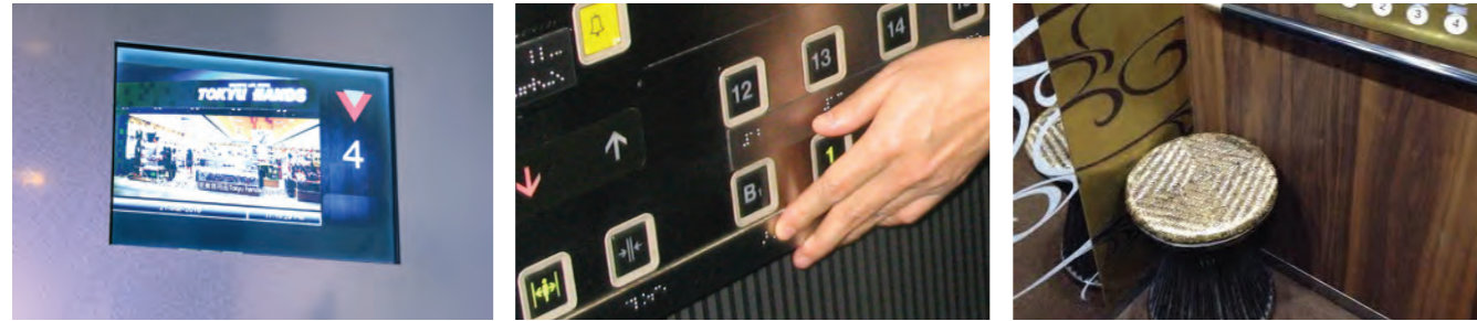
Photos (above): Wheelchair user manoeuvring out of the lift with the aid of mirrors and grab bars; seat within a lift; braille and tactile indicators on control buttons in the lift; visual information display system within the lift
